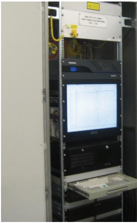
Fiber-optic control panel
